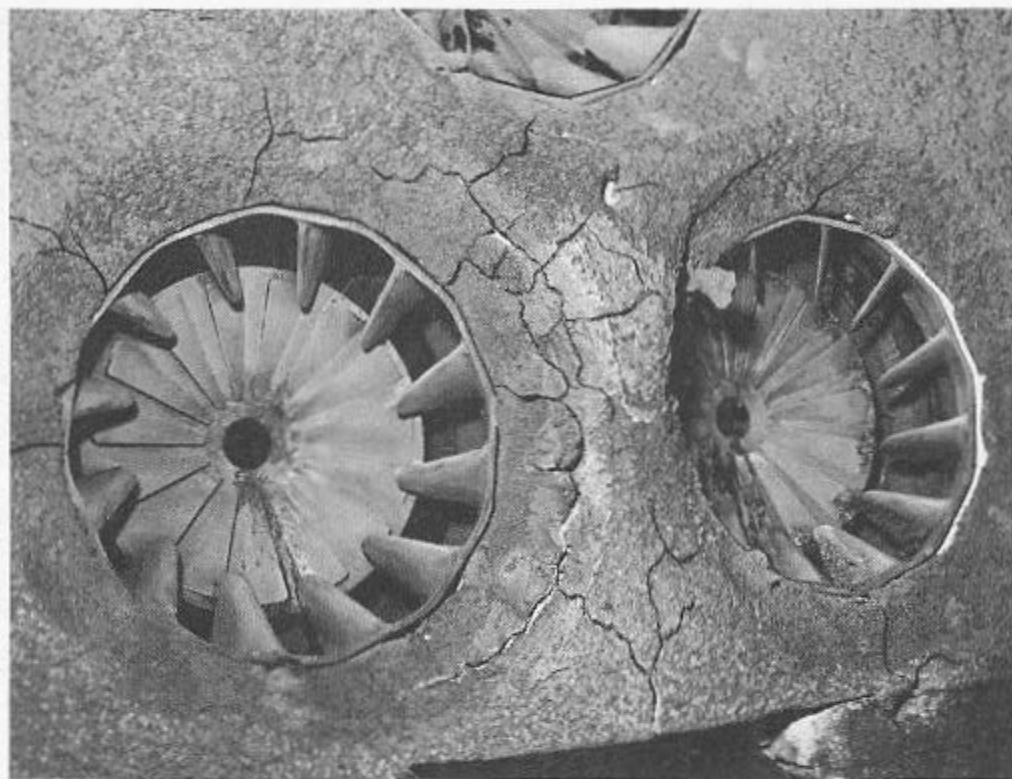
Figure 2-45.—Parallel cracks in burner front.
