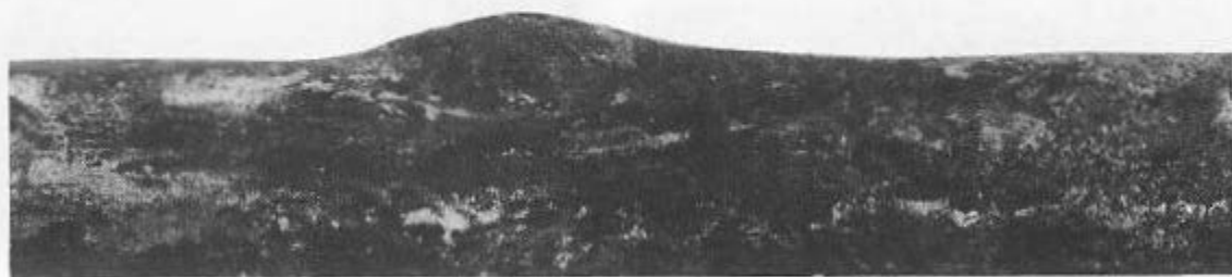
Figure 2-32.—Heat blister on fire row tube.
