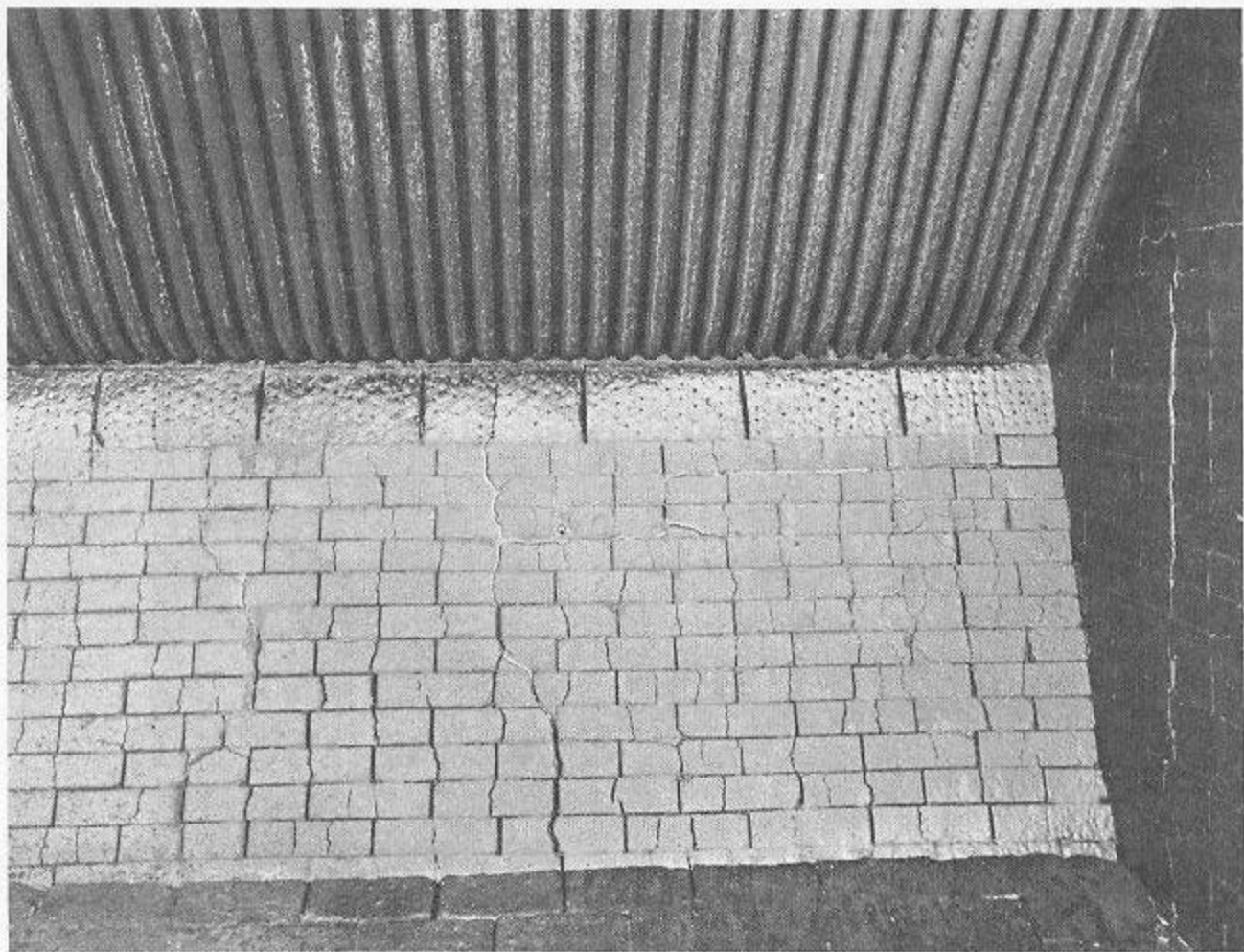
Figure 2-41.—Wall and sloping deck, showing excessive shrinkage of firebrick.
